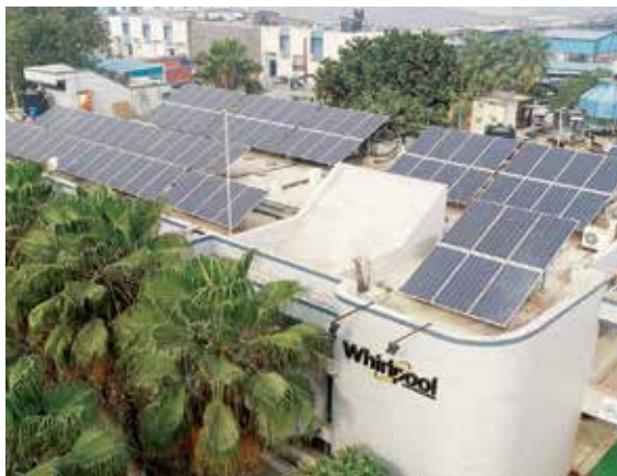
Solar panels installed at Faridabad factory
